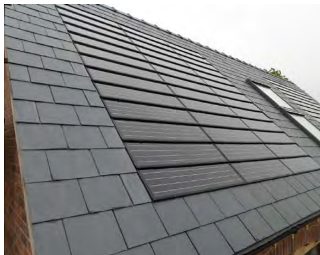
Figure 34: Integrated solar panels on slate roof.
